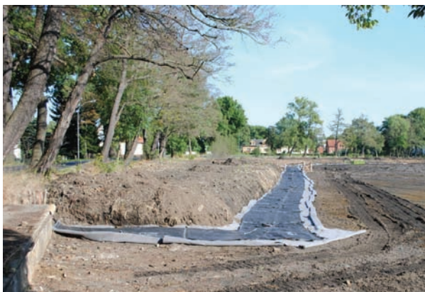
Fig 12. Placed non-woven and tubes in construction phase 2 before start of filling process
