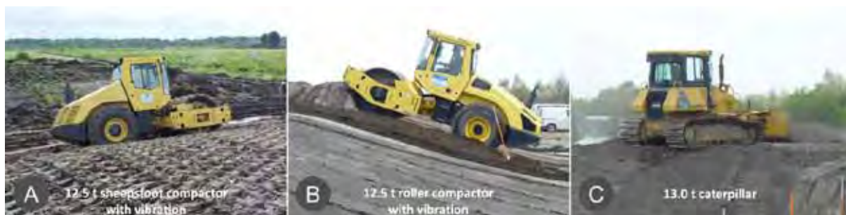
Figure 8. Three variations of compaction tested on the DredgDikes test dike in Rostock
